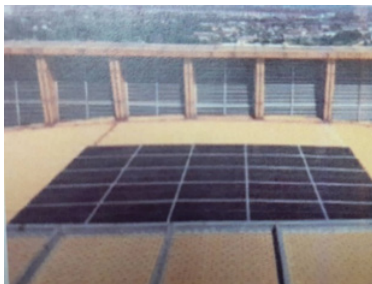
Solar Panels on the Roof of Navamindhrathiraj Building
